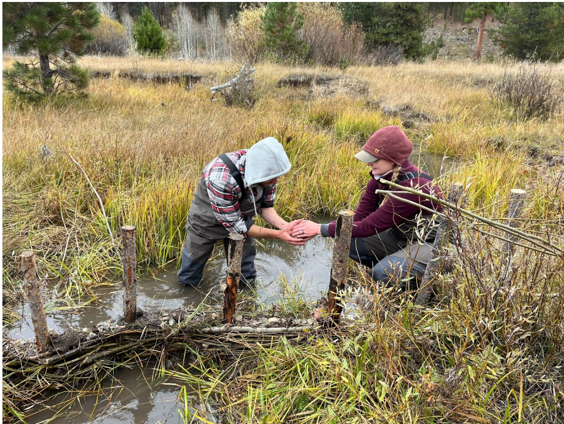
Volunteers wade, knee-deep, to complete the construction of a Beaver Dam Analogue (BDA)
